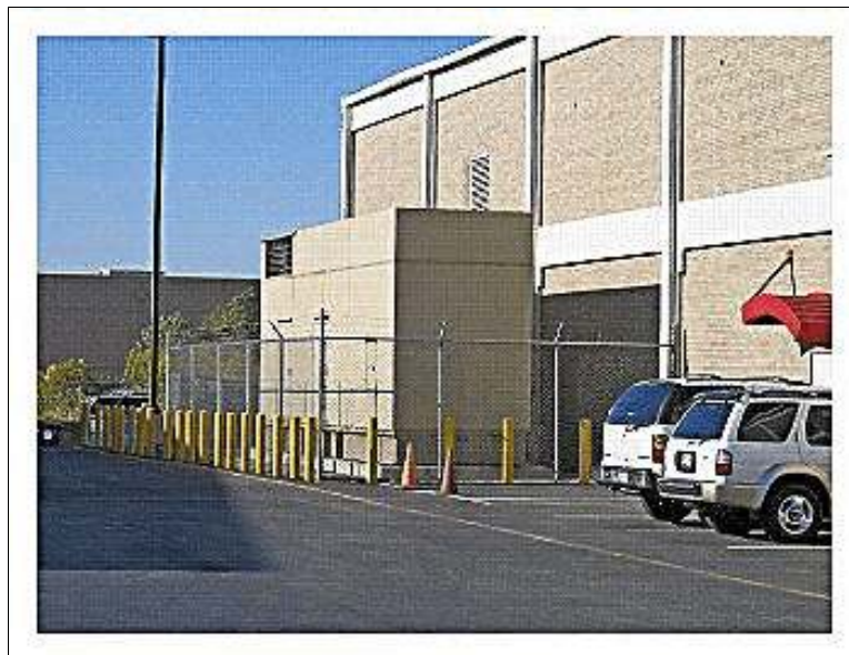
One of the two diesel generators
