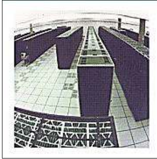
Inside the computer room
